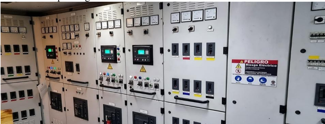
Figure 4. OPV ARC "20 de Julio" control panels
