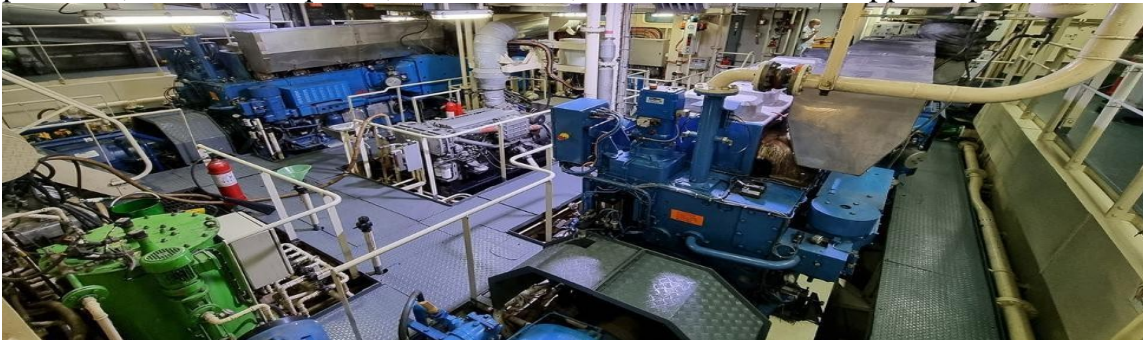
Figure 2. ARC OPV Engine Room "20 de Julio"
