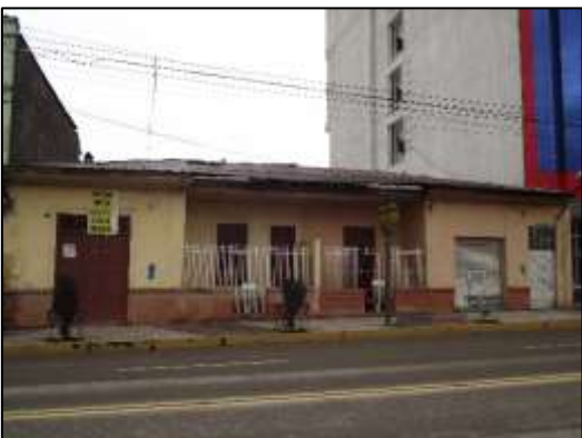
U-shaped typology in a state of deterioration (No. 789)
