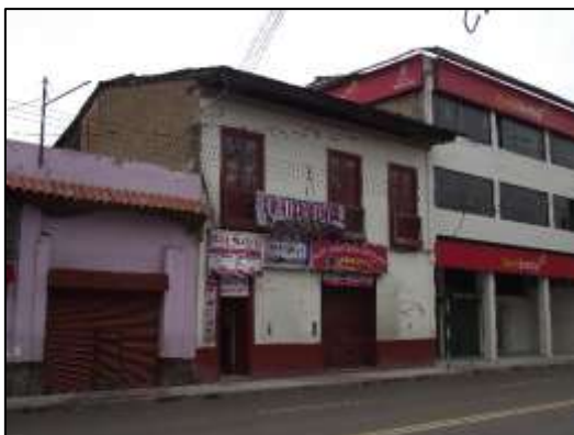
Figure 7: The change of use to which this urban framework is subjected is evident; which have determined a process of deterioration and degradation in their formal expression of
